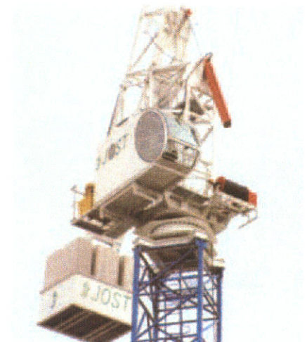
Above: Near King's Cross a Jost JTL 108.6 is rigged on a Peiner S 20 tower system. The detail view shows the unique luffing system consisting of a luffing ram (in red) and a compact electrohydraulic drive unit (in yellow). The hoisting winch (in red) is in front of the turntable
