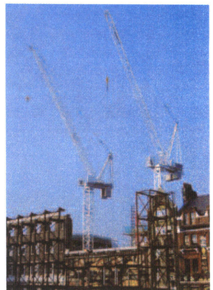
A Peiner SN 166 and SN 86, both with rope-moved ballast carriage, towering over the Aybrook apartment project at Blondford Street. Both models were developed with the UK crane market in mind. While the SN 166 is rigged with 40 m jib, providing a tip load of 4.3 tonnes, the SN 86 is rigged with 30 m jib for 3.15 tonnes tip load
